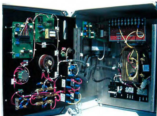
Watertank internal component view
