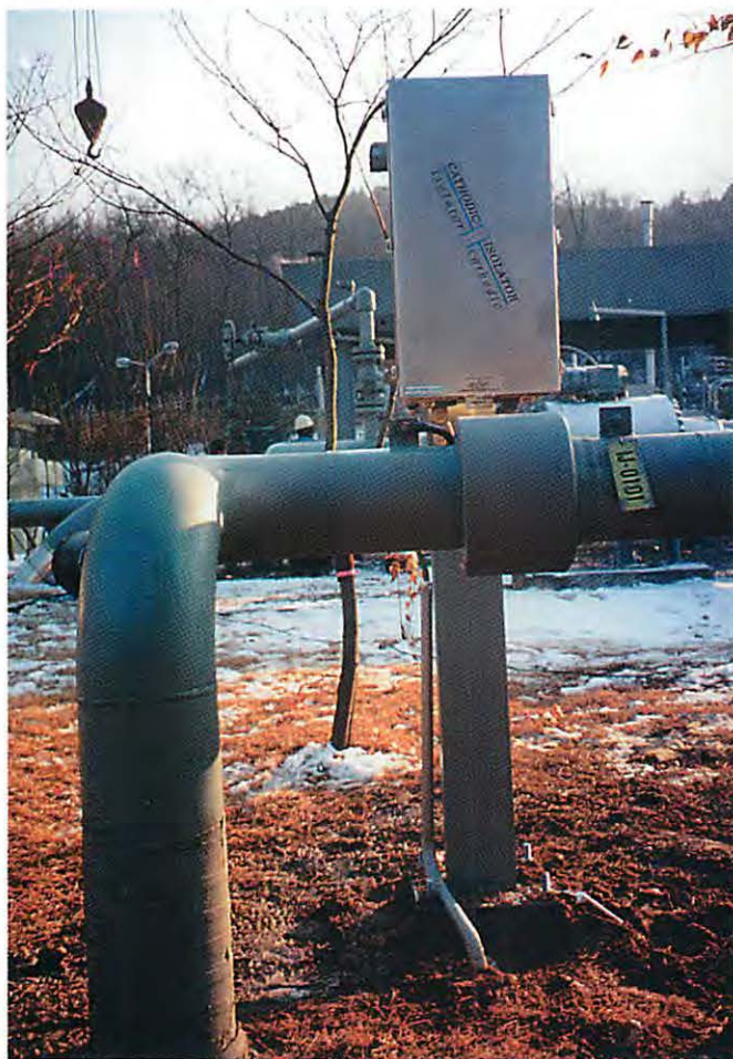
Protective equipment. Typical protective equipment installation across a monolithic isolating joint (and/or isolating flange).
